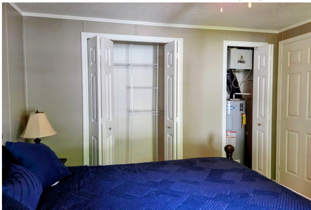
Closet + hot water heater & air exchanger
