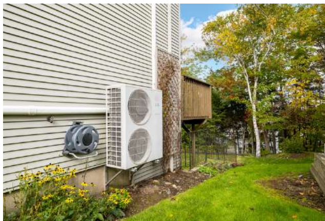
Side of house with mini-split fan
